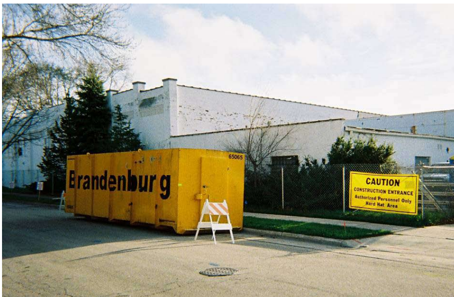
Cautionary sign at Cedar Creek Plant 2 site entrance
